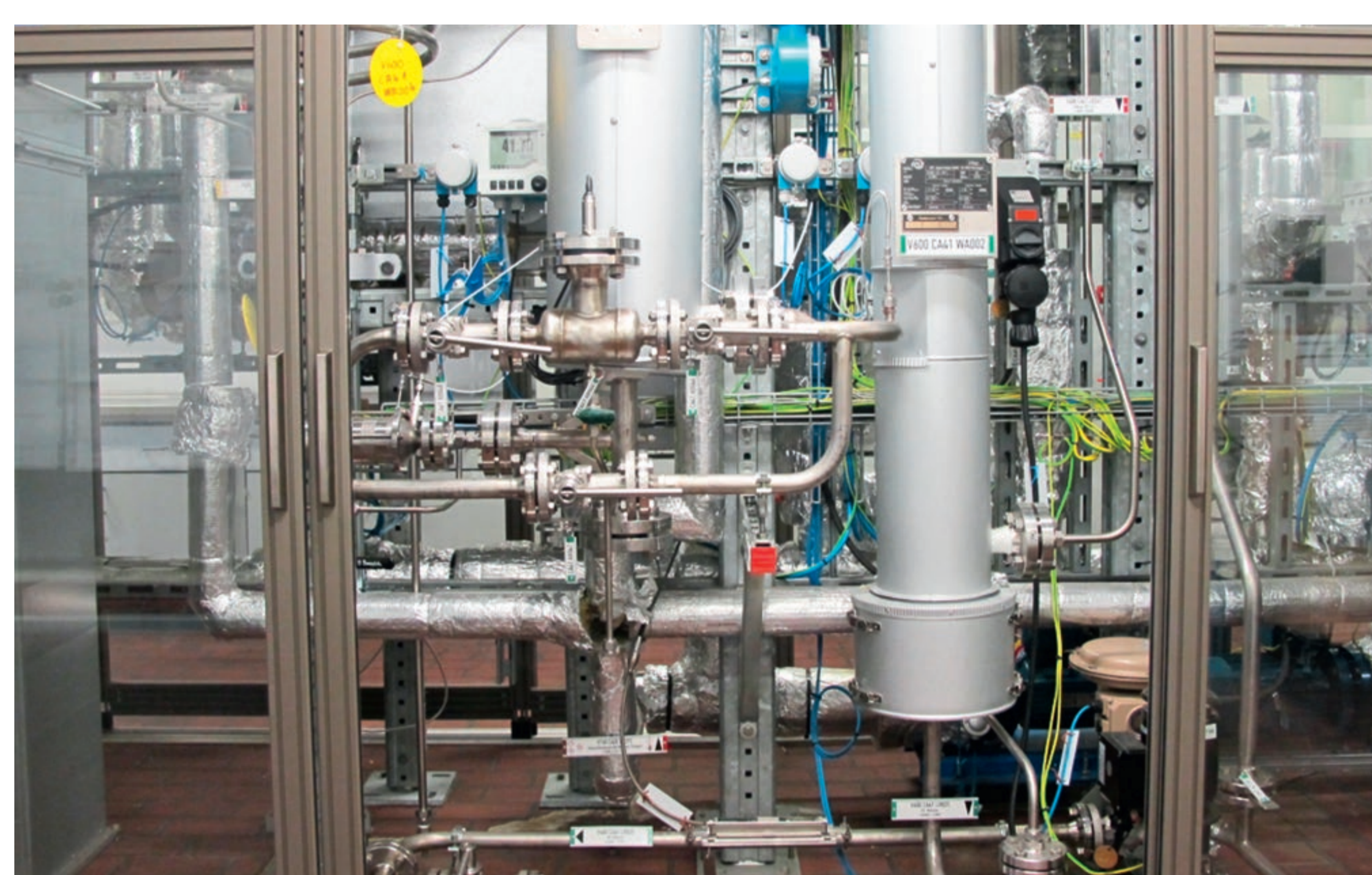
Miniplant for CO usage built up at Covestro.
